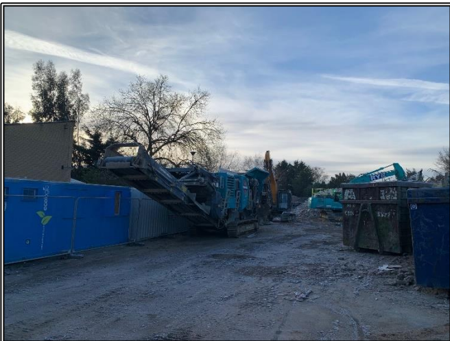
Crushing plant and access road
