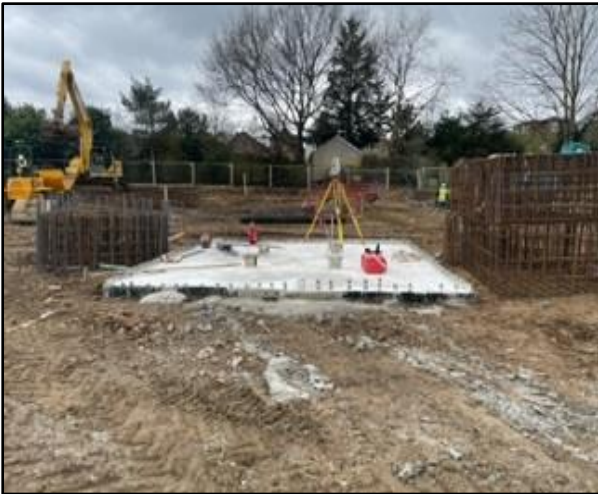
Tower Crane Base
