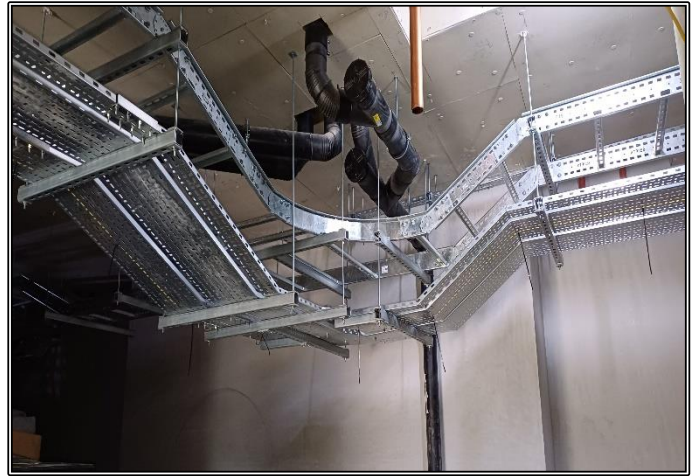
GF Plant Room Containment
